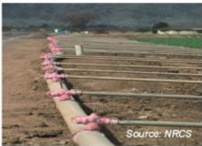
Mainline for handline sprinkler irrigation, Yuma, Az.
